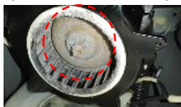
Fan get stuck by lint, and residue
